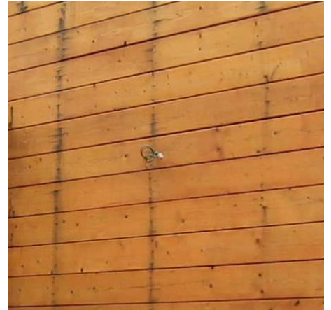
Stains around the attachment points due to corrosion.
